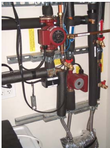
Picture 2: A 3-Way valve with Closed-Loop and DHW Pumps
